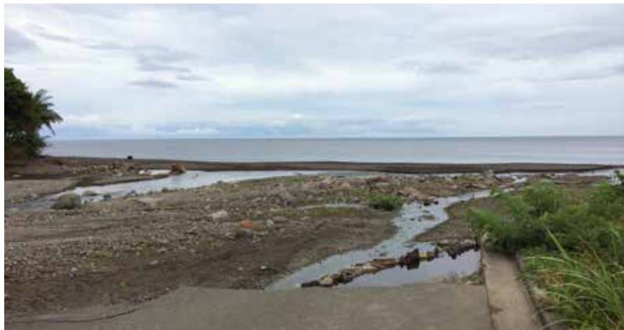
Leeward Highway near Richmond destroyed.
